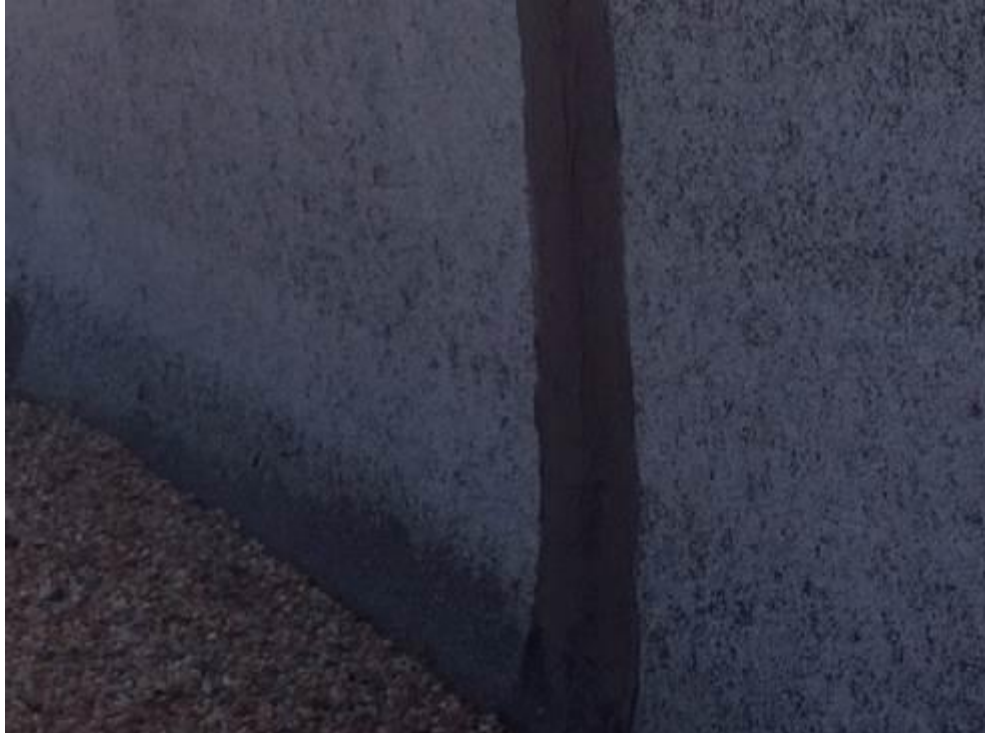
Roofing tar used on seams tested non-detect
