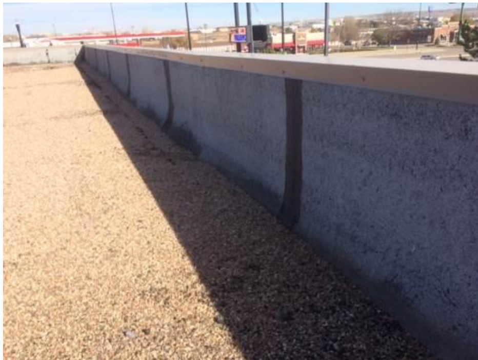
Tar and gravel base material and rolled roofing on parapet walls both tested non-detect for asbestos
