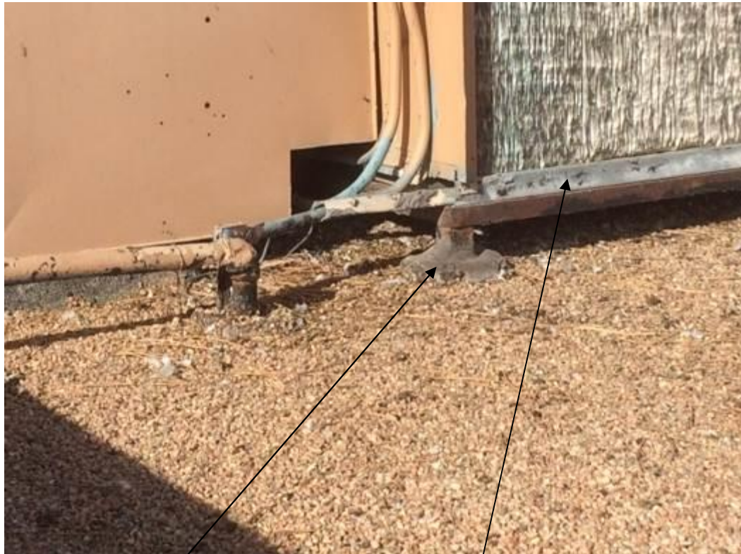
Tar on HVAC unit supports and associated gray sealant both tested non-detect for asbestos
