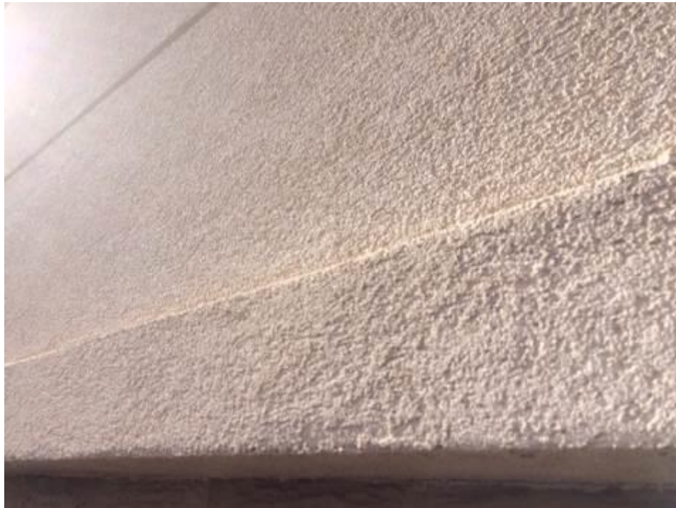
Stucco plaster on eastern elevation tested non-detect
